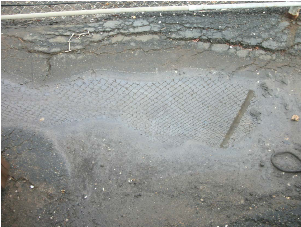
Photo #2: Staining of concrete near to the office to the west of the salt dome
