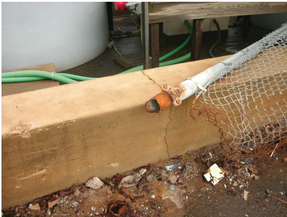
Photo #4: Crack in secondary containment around ASTs
