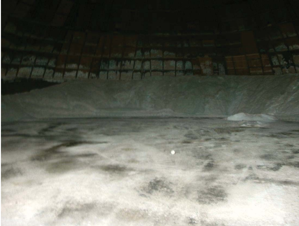
Photo #1: Minor staining of floor inside salt dome, assumed to be caused by salt
