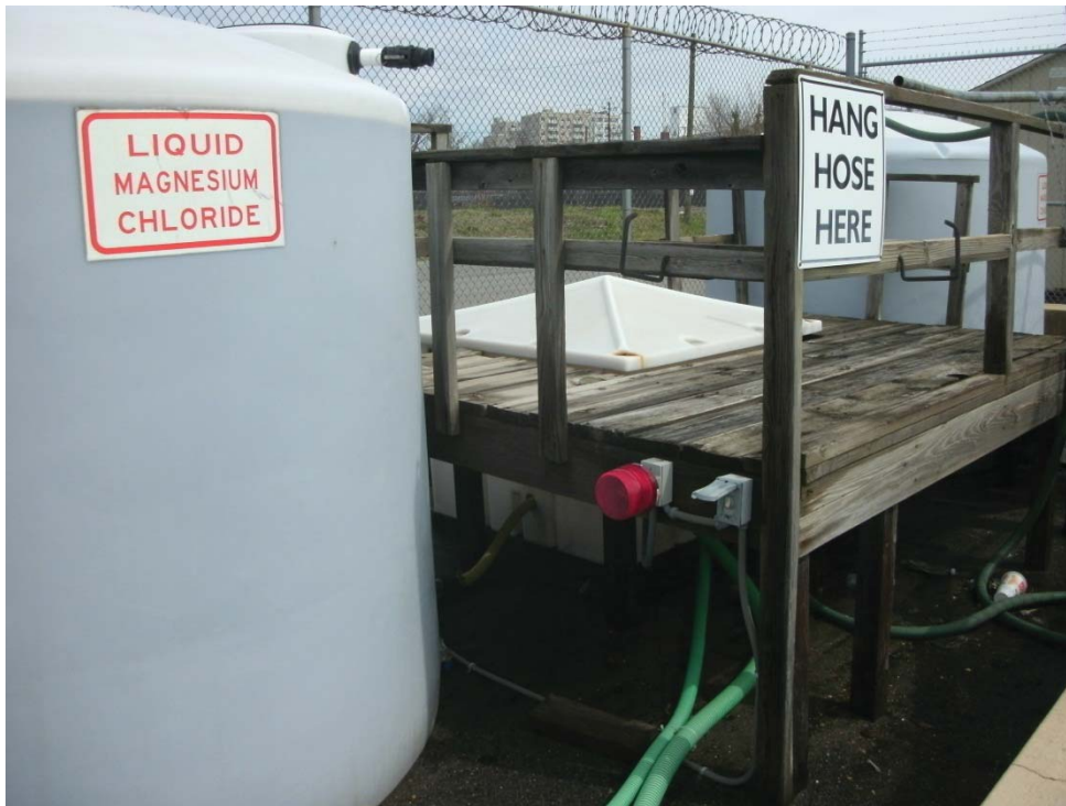
Photo #3: Magnesium chloride tank within secondary containment
