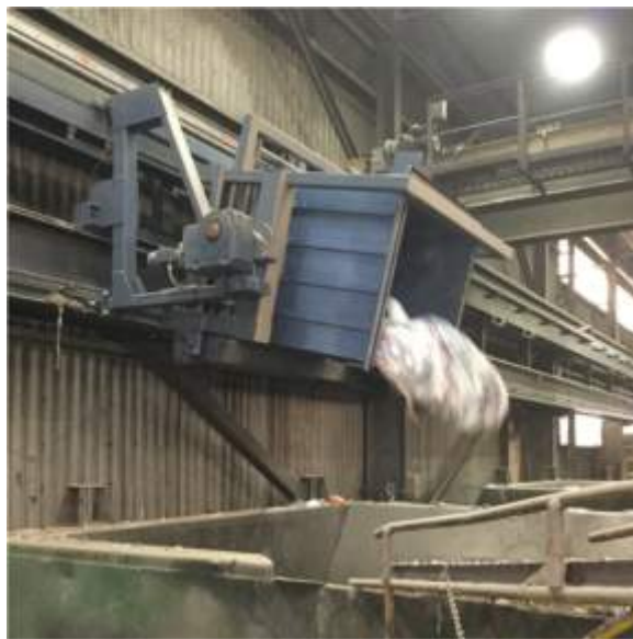
Figure 9 - WFS Dumping mechanism feeding MWC feed chute
